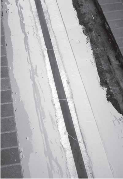
▲ A close up of the RedLINE expansion joint encapsulated in liquid membrane.
