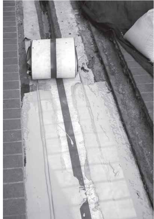
▲ The RedLINE being encapsulated on the top surface in a liquid membrane.
