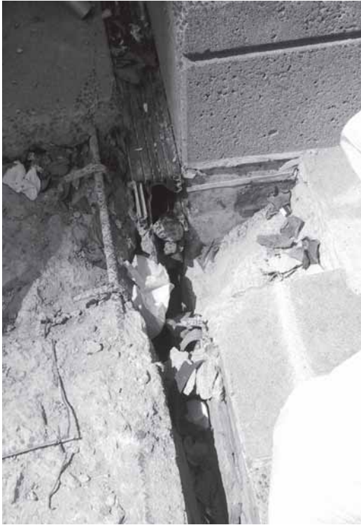
▲ The expansion joint cavity exposed at a detail, prior to membrane application.
